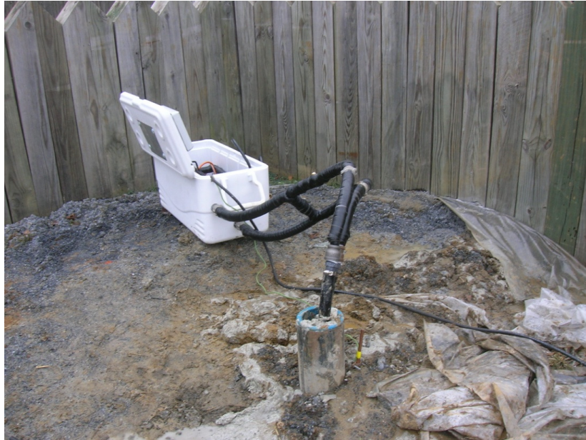
Figure 8 Test box connected to Borehole Heat Exchanger
